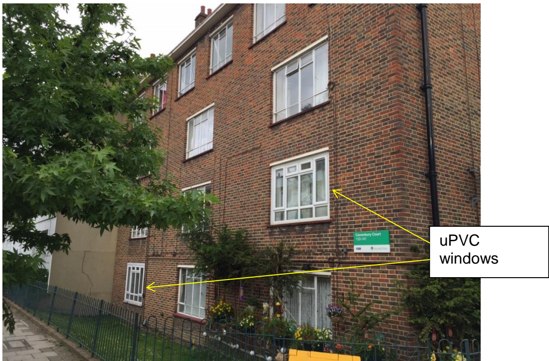
IMAGE 2 The west elevation of the building, it is noted that some uPVC windows have been installed on this elevation and the south elevation (see image 4) without planning consent.
