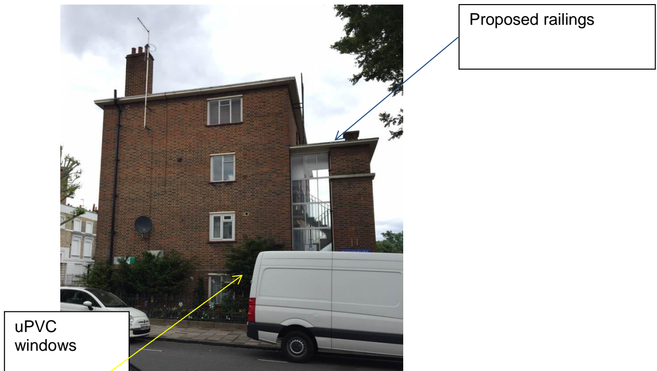
IMAGE 4: The south elevation of the building on Hawes Street, the railings will be installed at the top of the stairwell.
